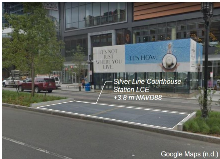
Figure 4. Sample Lowest Critical Elevation (LCE), a ventilation shaft at street level directly above Courthouse Station along the MBTA Silver Line in South Boston (Google, n.d.)
